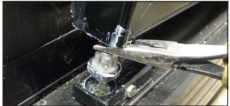
Fig. 7. An assistant lifting the torsion rod from the torque master hole while the technician lifts the door.
