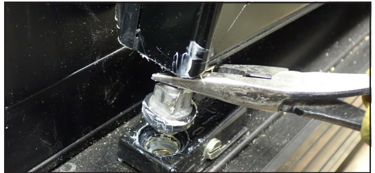
Fig. 7. An assistant lifting the torsion rod from the torque master hole while the technician lifts the door.
